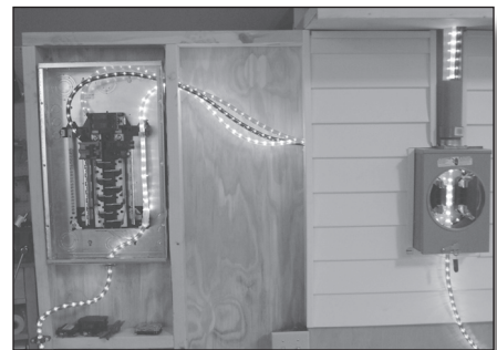
Figures 2 and 3 (above and left). Components of the electric distribution system are displayed and controlled to provide a better understanding of the route electricity takes in its journey to your home.
